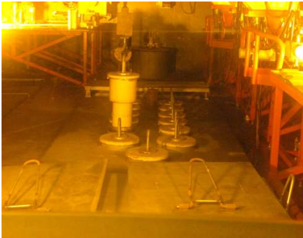
Figure B5: The Storage Pits at LEPI for Irradiated Experimental Fuel Rods and Fragments
